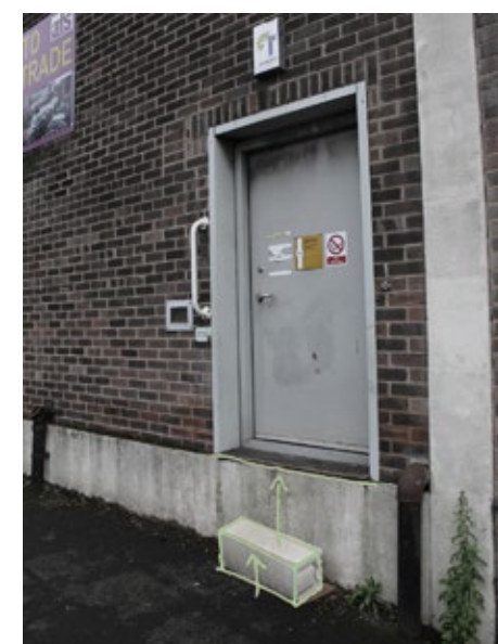
Large drops on some doors, hard to access
